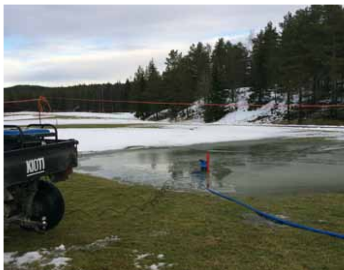
Picture 15. Removal of melting water from green with generator and mobile pump at Grønmo GC. Photo: A. Fern.
